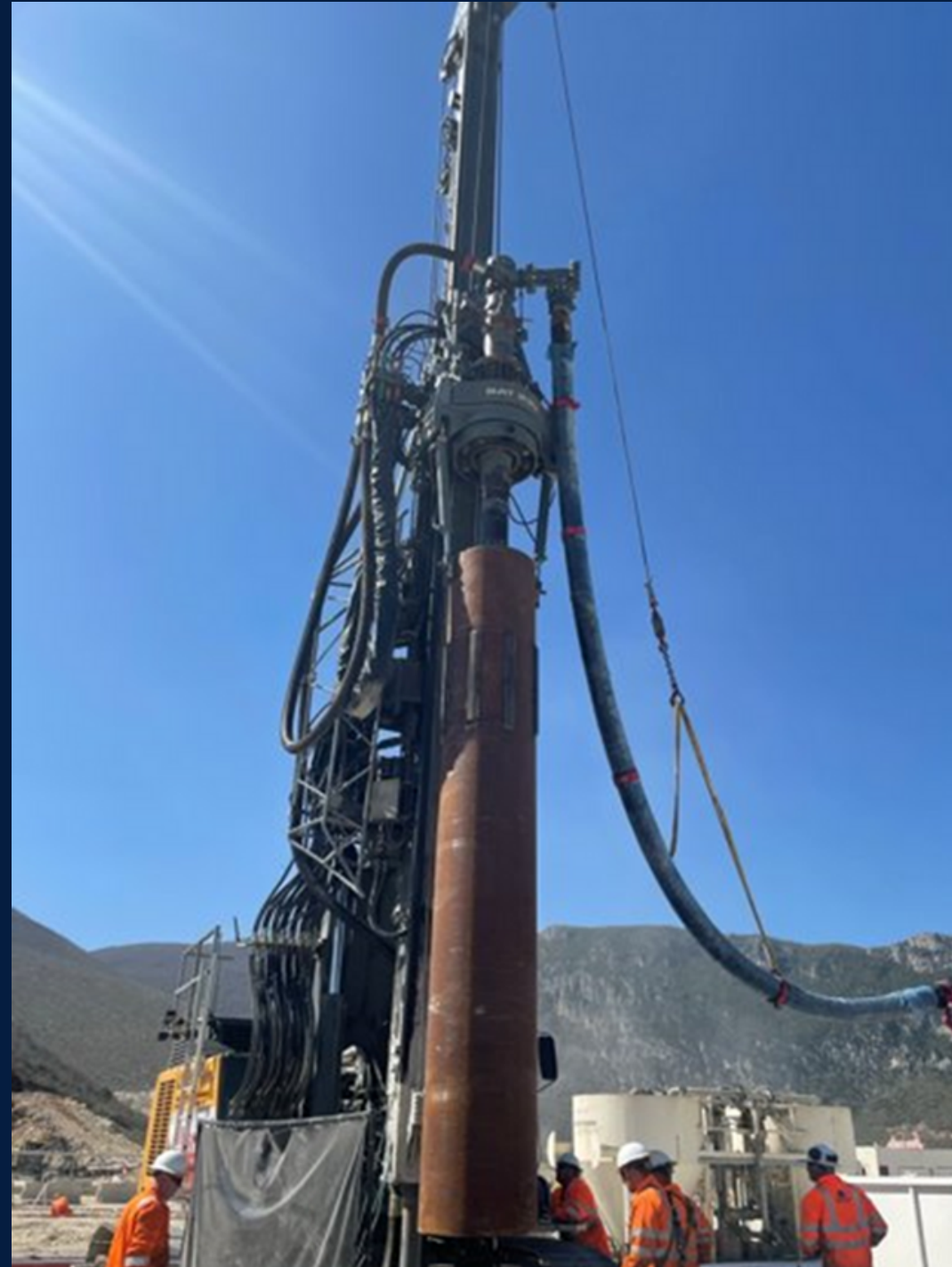
LB 20 successfully drilled a 43" conductor well down 377' in hard rock Albania. Used a casing advancement system to install casing.
