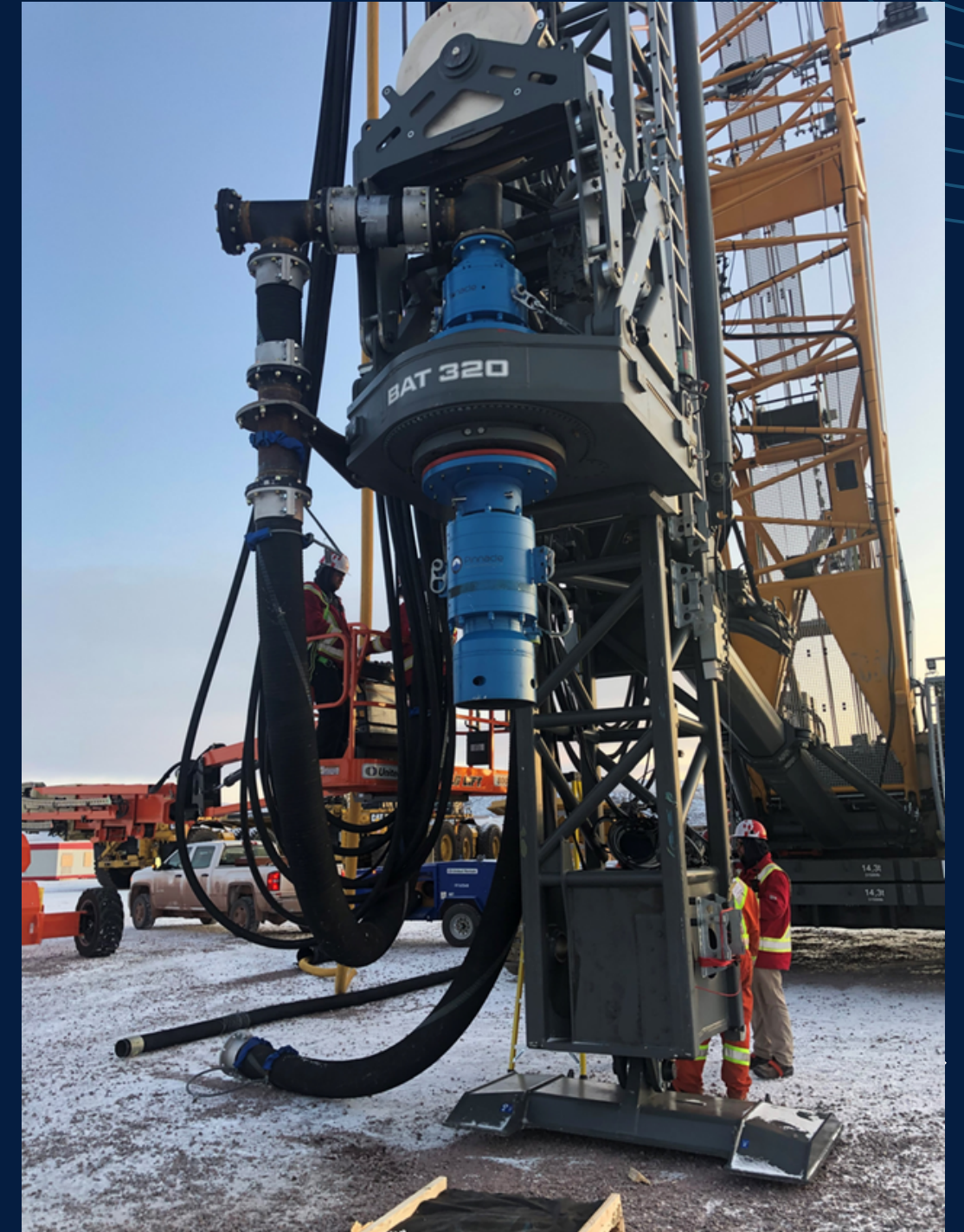
Installation on BAT320 mounted on Liebherr lead with 300Ton crane for project in North West Territories (CAD) drilling single pass in permafrost
